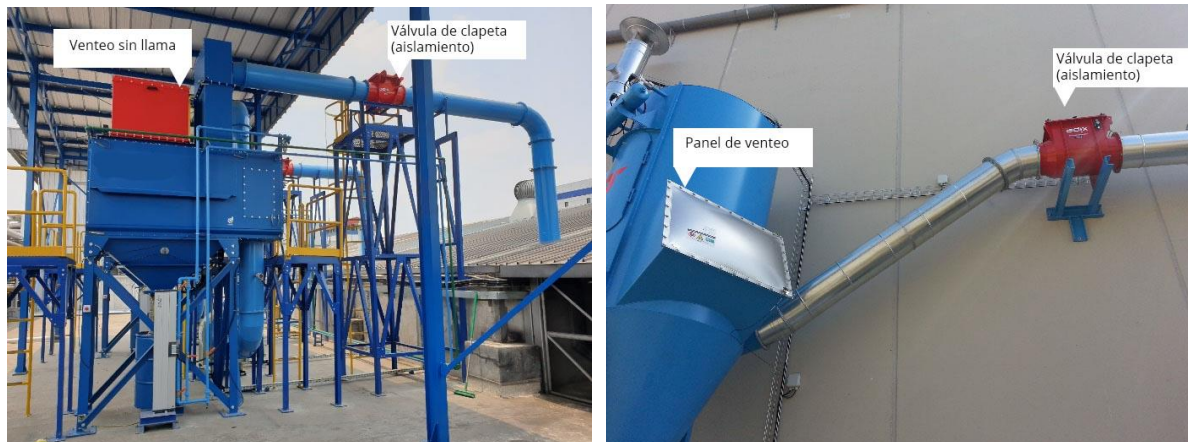
Fig. 5. Baghouse protection systems
